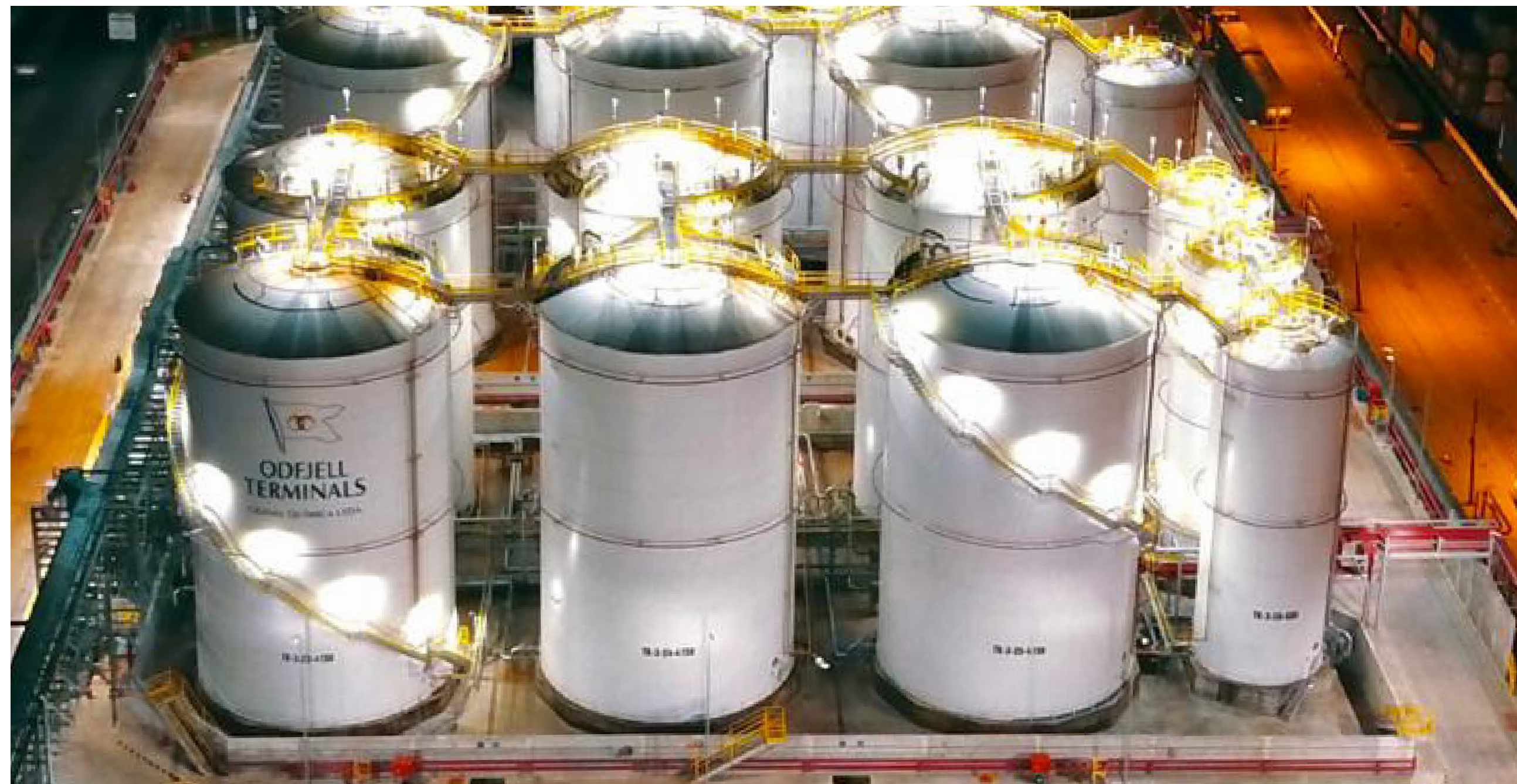
Terminal Santos, led lighting in internal roads, tanks, catwalks, loading platforms and offices.
